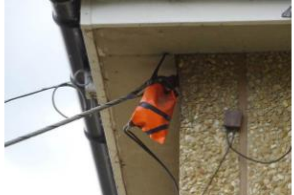
S56 – 3 Upper Park Road, Nailsworth. Overhead electric cables
