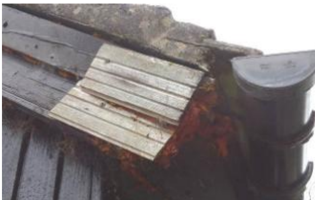
T23 – 6 The Knoll, Uley. Outbuilding roof, poor repair to verge fascia at eaves
