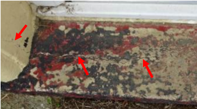
S31 – 51/52 Mankley Road, Leonard Stanley. Crack on door step extending up onto reveal
