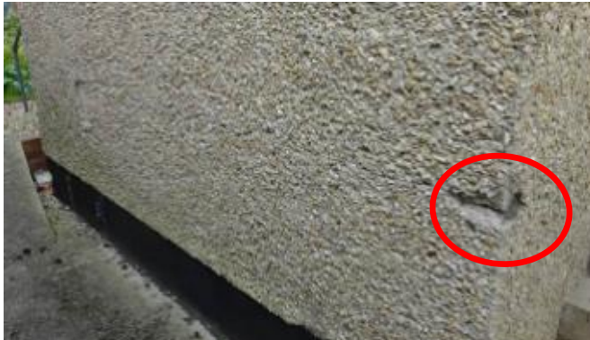
S43 – 6 Upper Park Road, Nailsworth. Side extension, cracking at dpc level
