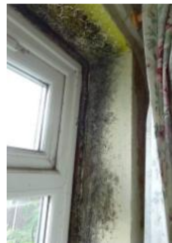
S30 – 39 Mankley Road, Leonard Stanley. Mould in window reveal at head (one of many windows affected)
