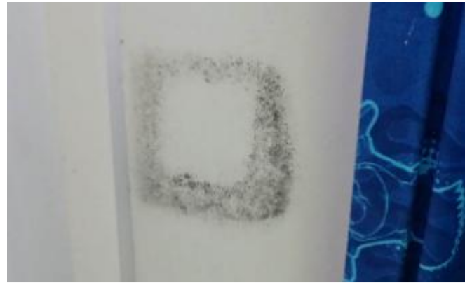
S20 – 12A Lawnside, Forest Green, Bedroom mould to left of window mid height
