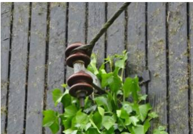
T11 – 32 Barrs Lane, North Nibley. Incoming mains electrics on side elevation
