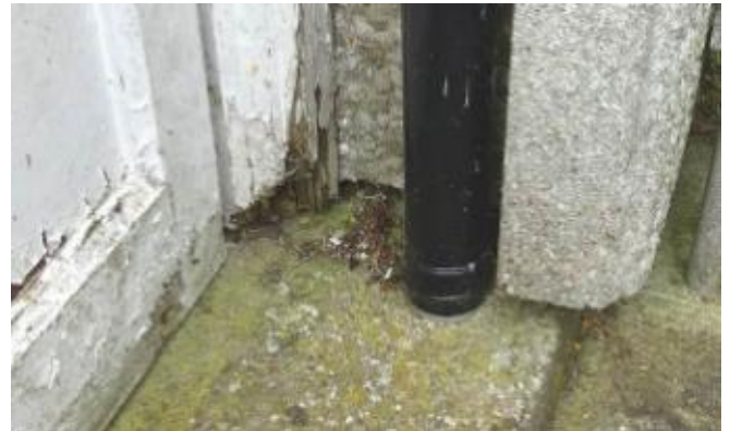
Q14 – Example of porch door close to rainwater downpipe & corner (problem with EWI)
