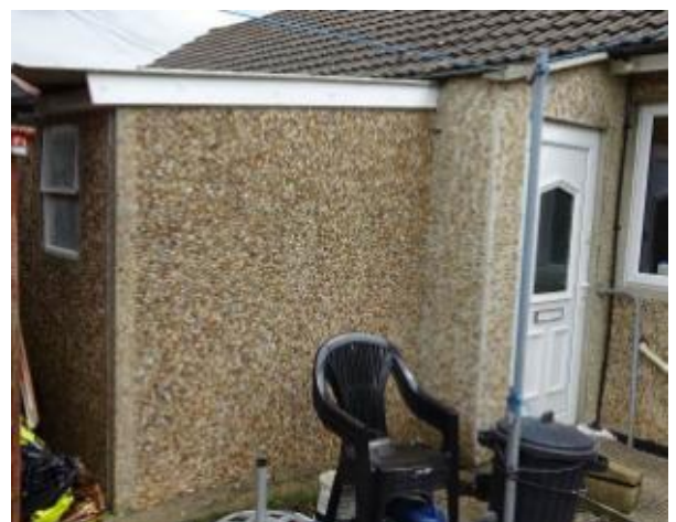
S36 – 38 Glebe Road, Minchinhampton. Outbuilding of Reema panel construction jointed to bungalow
