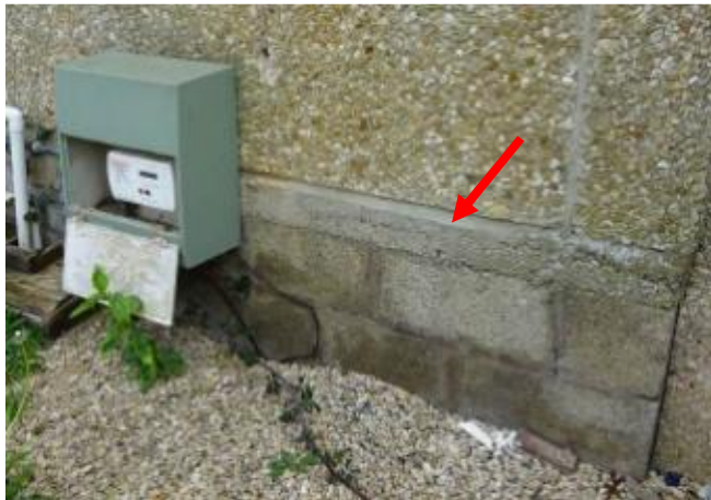
S45 – 6 Upper Park Road, Nailsworth. Rear corner main house. Cast in-situ concrete (arrowed) & blockwork suggests underpinning
