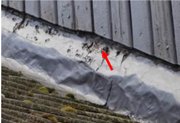
T19 – 3 Bushey Beeches, The Camp. Flashing at junction of Outbuilding & main house. Original flashing covered by “flashband” type repair, starting to disintegrate (arrowed)
