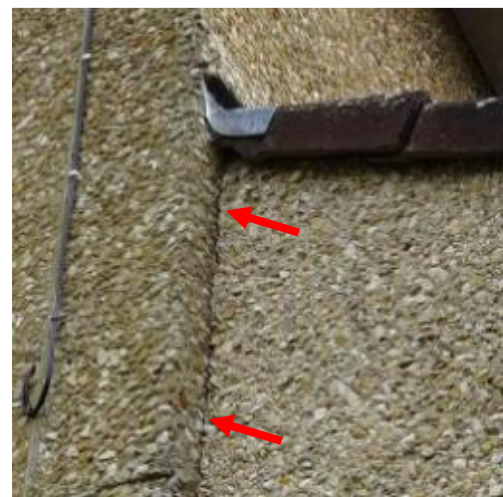
S40 – 6 Upper Park Road, Nailsworth. Cracking at junction of side extension & main house
