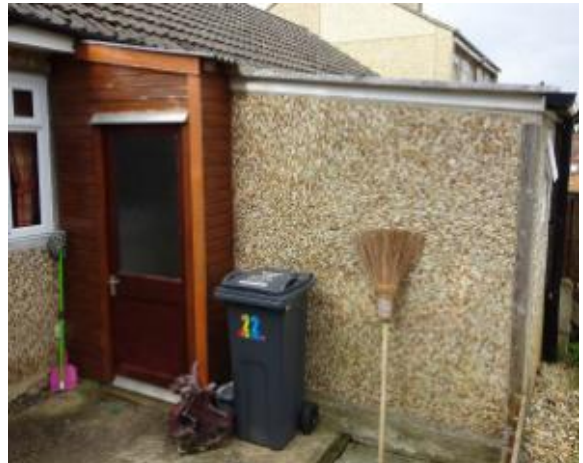
S58 – 22 Willow Road, Stonehouse. Outbuilding joined to the bungalow (note: Outbuilding is of Reema panel construction)
