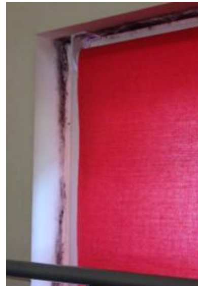
S22 – 12A Lawnside, Forest Green, Bedroom 2 mould on window reveal & head
