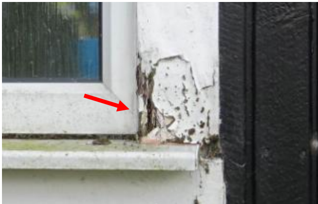
T33 – 3 Mount Pleasant, Wotton-Under-Edge. Side, rot to window architrave
