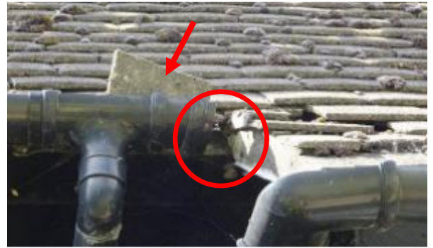
T38 – 7 Mount Pleasant, Wotton-Under-Edge. Rear slipped tiles (arrowed) & gap between gutter & roof (circled)
