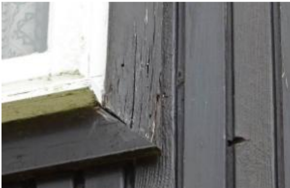
T15 – 3 Bushey Beeches, The Camp. Front first floor window, rot to architrave
