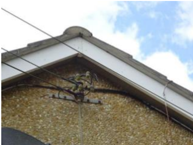
S57 – 6 Upper Park Road, Nailsworth. Overhead electric cables
