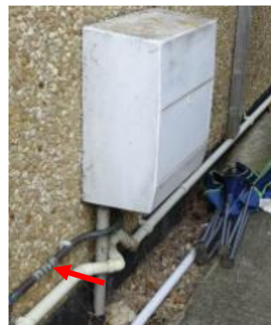
S34 – 39 Mankley Road, Leonard Stanley. Gas meter box & pipework
