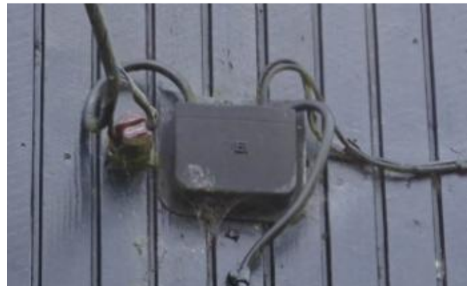
T34 – 3 Mount Pleasant, Wotton-Under-Edge. Incoming mains electrics on side elevation
