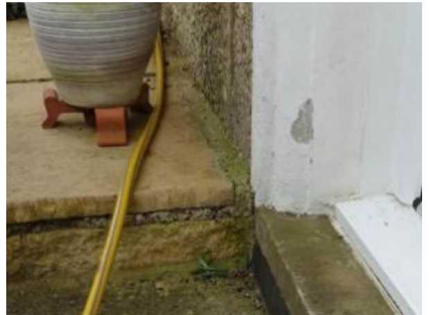
S28 – 18 Lawnside, Forest Green, paving to left of front door too high
