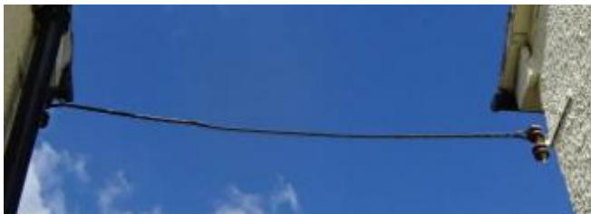
P9 – Typical overhead power supply cables between buildings (this one at 14 Mosley Cresnet, Cashes Green)
