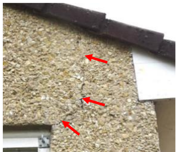
S42 – 6 Upper Park Road, Nailsworth. Cracking above door
