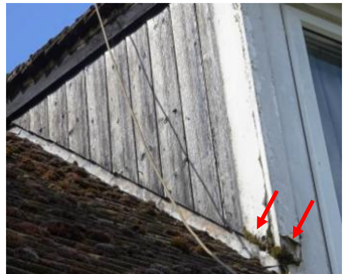
T40 – 7 Mount Pleasant, Wotton-Under-Edge. Rear, poor timber to dormer side, and architrave rotten near roof tiles (arrowed)
