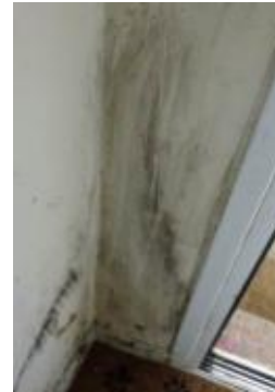
S32 – 51/52 Mankley Road, Leonard Stanley. Mould on external wall at bottom of stairs to first floor flat.
