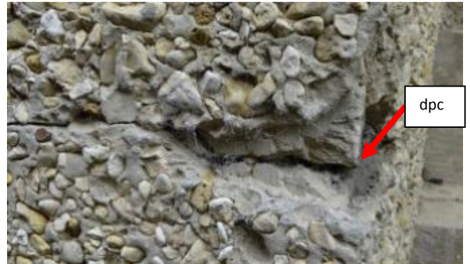
S44 – 6 Upper Park Road, Nailsworth. Side extension, cracking at dpc level detail
