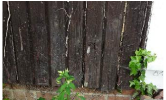
T28 – 6 The Knoll, Uley. Rear, example of rot & split outer boards near party wall
