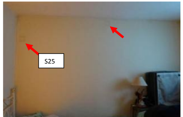
S24 – 45 Lawnside, Forest Green, bedroom gable wall, two small square areas of staining (arrowed). Photo S26 is to the right side.
