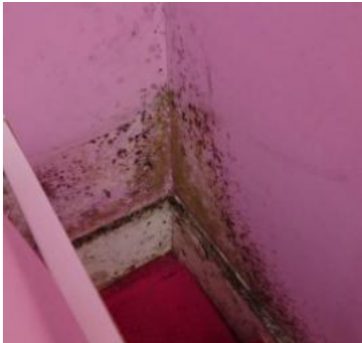
P7 – 14 Mosley Cresnet, Cashes Green, mould in front ground floor room used as bedroom
