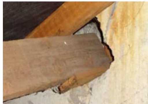
S52 – 3 Upper Park Road, Nailsworth. Roof purlin at party wall. Hole through to other side of wall, risk of fire spread.
