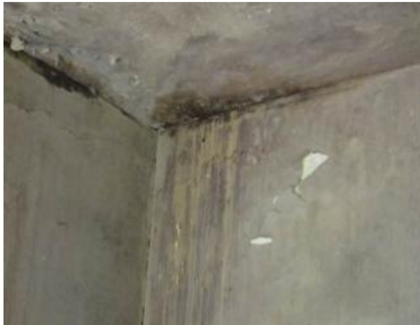
S69 – 31 Victory Road, Whiteshill. Side extension mould & damp ingress staining in front corner
