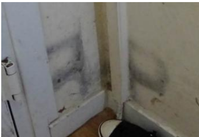
S17 – 12A Lawnside, Forest Green, Hall mould in square shapes on front & alleyway walls
