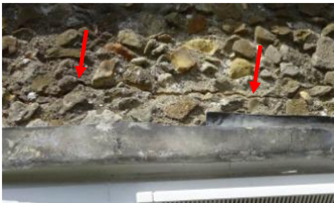
S63 – 31 Victory Road, Whiteshill. Side extension cracking above window detail
