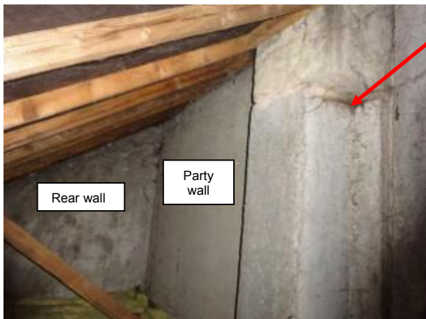
S53 – 6 Upper Park Road, Nailsworth. General view in loft towards rear & party wall
