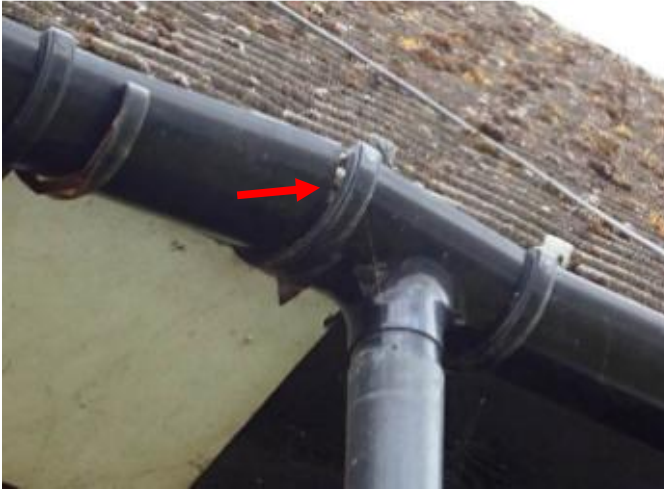
T7 – 32 Barrs Lane, North Nibley. Front gutter disconnected at downpipe bracket (arrowed)
